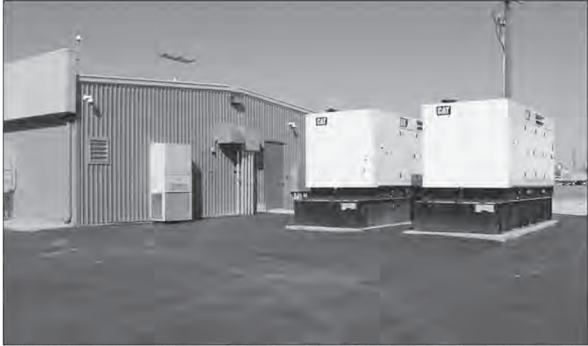
Powerful backup generators are ready in the event of a power outage.
